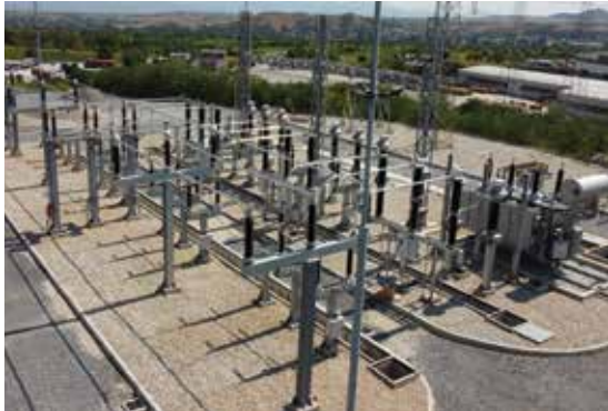
Private Substation 110/10kV
