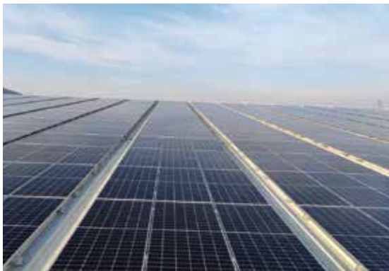
Rooftop PV Plant
